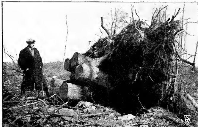
In construction work a deal of stump-pulling is often necessary; above shows the type of stump that the "K" hand stump-pulling outfit took care of at Canoebrook, N. J. Stump & Walter Co.'s seeds were used on this course.
