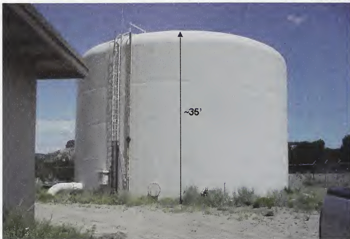
Figure 9. Photograph of existing steel water tank at Booster Station 1.
