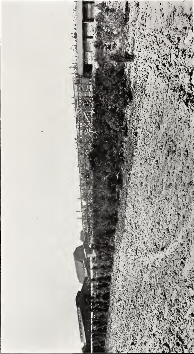
Framework of building, in course of construction, covering a portion of our packing grounds, thus affording requisite protection to trees and shrubs from sun and wind. Forcing beds under canvas, packing and storage barns in the distance. Notice some of our employees cultivating and thinning block of evergreens.
