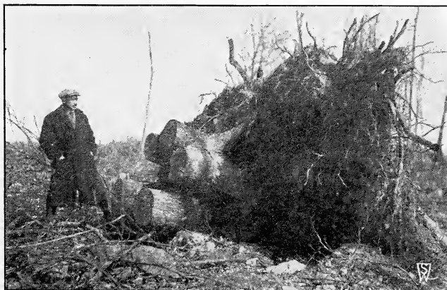
In construction work a deal of stump-pulling is often necessary; above shows the type of stump met with at Canoebrook, N. J. Stumpp & Walter Co.'s seeds were used on this course.
