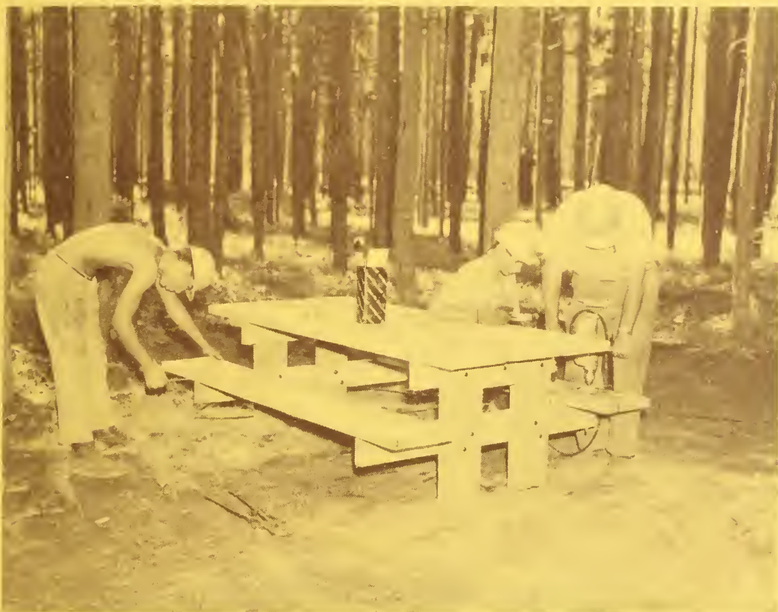
The U.S. Forest Service Operation Outdoors calls for widespread construction and improvement of campgrounds and picnic areas to meet the accelerating recreation demand. (Targhee National Forest)
