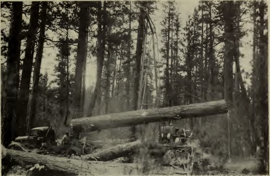
Figure 8. Loading a 32-foot log with the Le Tourneau industrial crane. Mobile loading equipment, making frequent moves to new landings feasible, is essential to the Blacks Mountain method of cutting .
