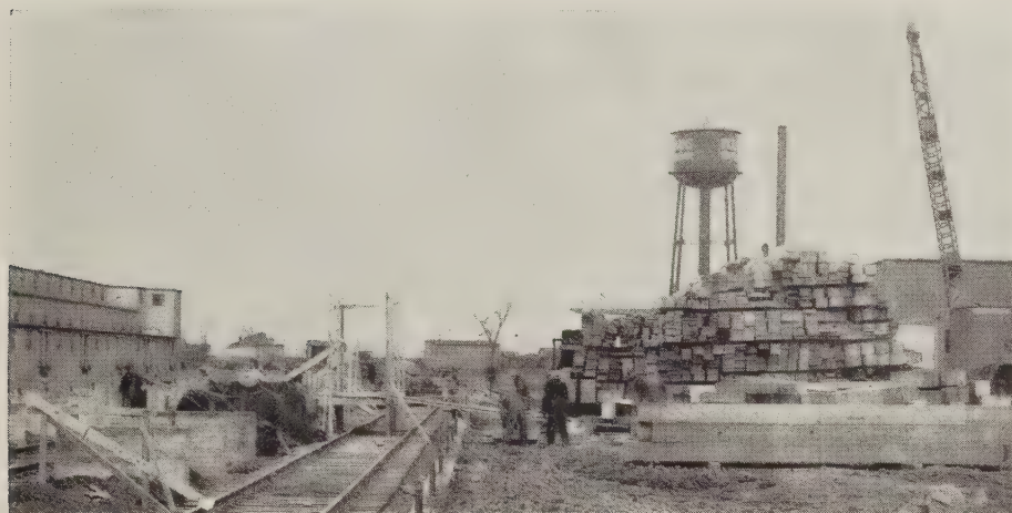
☆ Compare that stack of lumber with the height of the men constructing the new loading shed at the Eastern States Mill in Buffalo and you get an idea of what a whopping big roof it takes to cover 39 freight cars.
