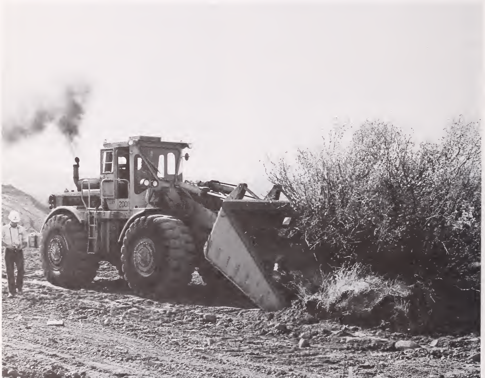
Figure 3.--Dryland sodder preserves topsoil and its vegetation for later replacement on reshaped spoil materials.
