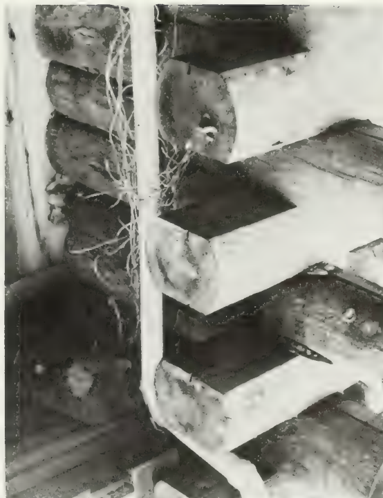
Fungus fruiting bodies on several logs and in the corner indicate advanced decay in a 5-year-old log house. Roof runoff onto log ends encourages decay.
