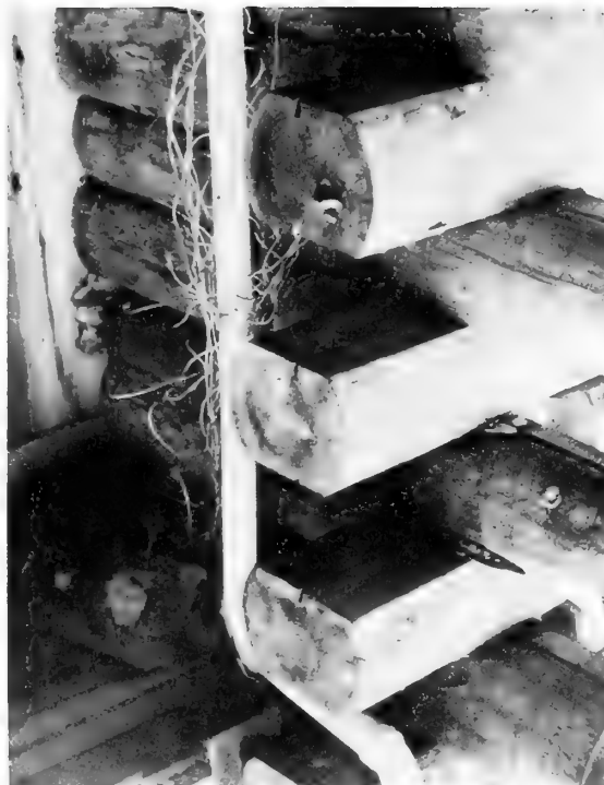
Fungus fruiting bodies on several logs and in the corner indicate advanced decay in a 5-year-old log house. Roof runoff onto log ends encourages decay.
