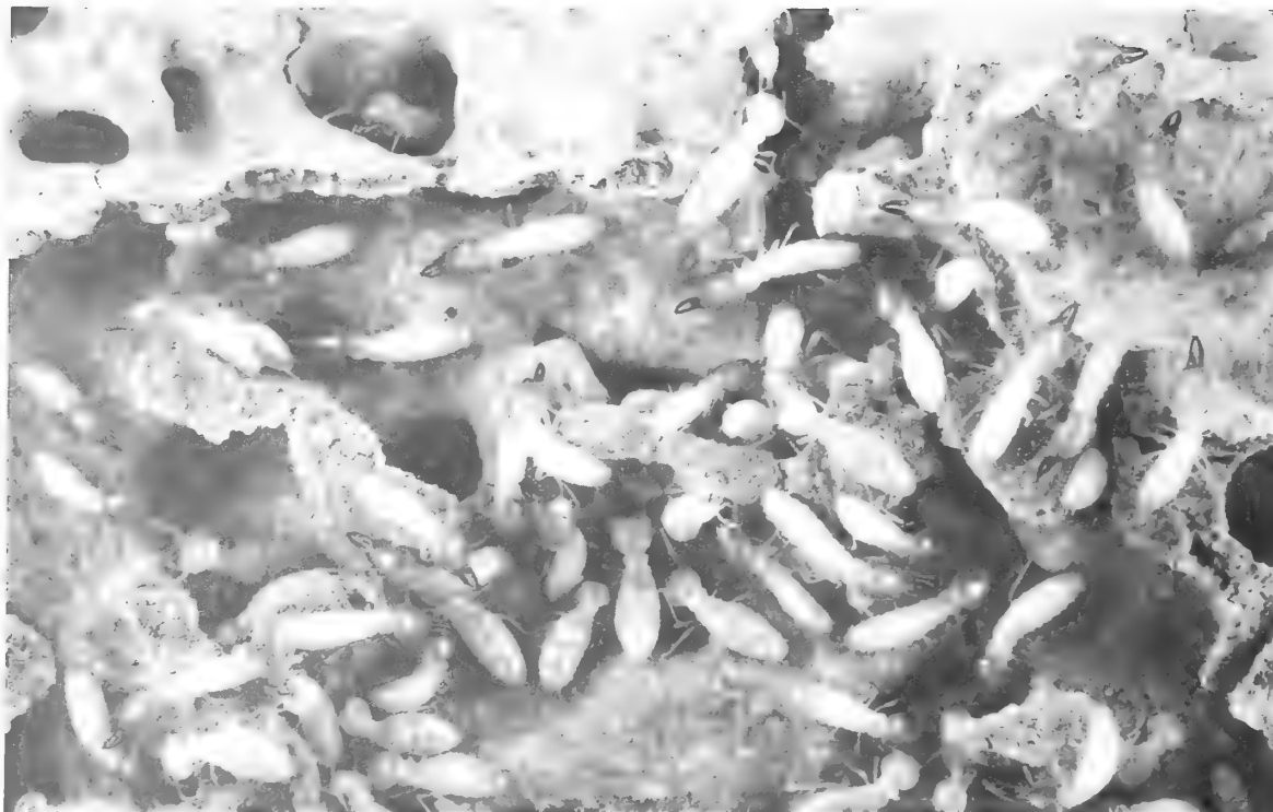
Without control, subterranean termites can make short work of wood on or near the ground.
