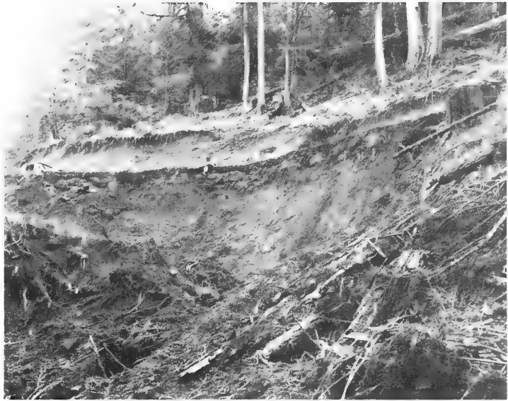
Figure 6.--Massive roadfill failure caused by blockage of road drainage ditch.
