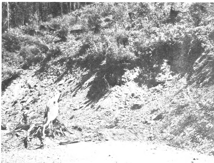
Figure 3.--Backslope failure in an area of soil derived from andesite colluvium.
