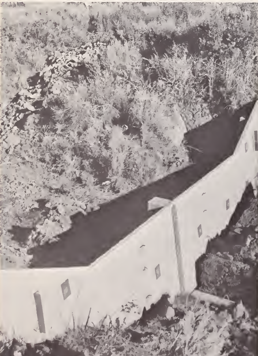
Figure 6.-- Looking at the upstream face of the completed dam before it is backfilled.
