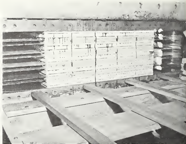
Figure 3.--Five panels were assembled and pressed at one time. Note squeeze out of glue.
