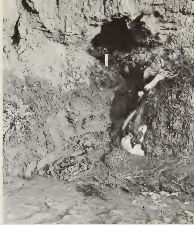
Figure 11.--The outlet of soil pipe 3, located about 4 feet above the gully bottom, during the spring snowmelt of 1963. Recent pipe flow, exhausted by lack of snow outside of the gully, caused the erosion on the gully side slope below the outlet. The increased slope gradient below the pipe outlet raised the load-carrying capacity of the pipe flows and thus made this erosion possible. Snows in the headwaters still feed the flow in the gully. Note the wetting of the gully side slope to the approximate elevation of the pipe outlet. Ruler is 4 inches long.
