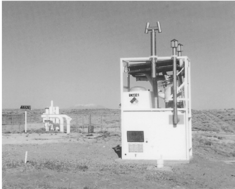
Figure 10.3 Installation of a closed cycle vapor turbogenerator on a gas pipeline in the western United States. (Courtesy of Ormat.)
