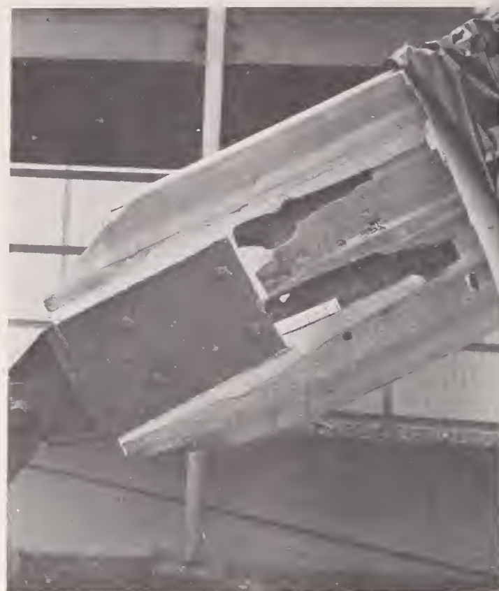
Figure 46. Decay in exposed laminated arch.
