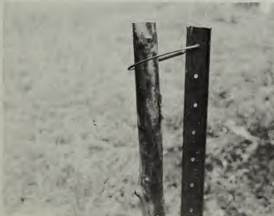
CLOSEUP OF NO. 9 WIRE THROUGH METAL POST AND AROUND STAY. SHOWN IS A NICROPRESS SLEEVE SPLICE
