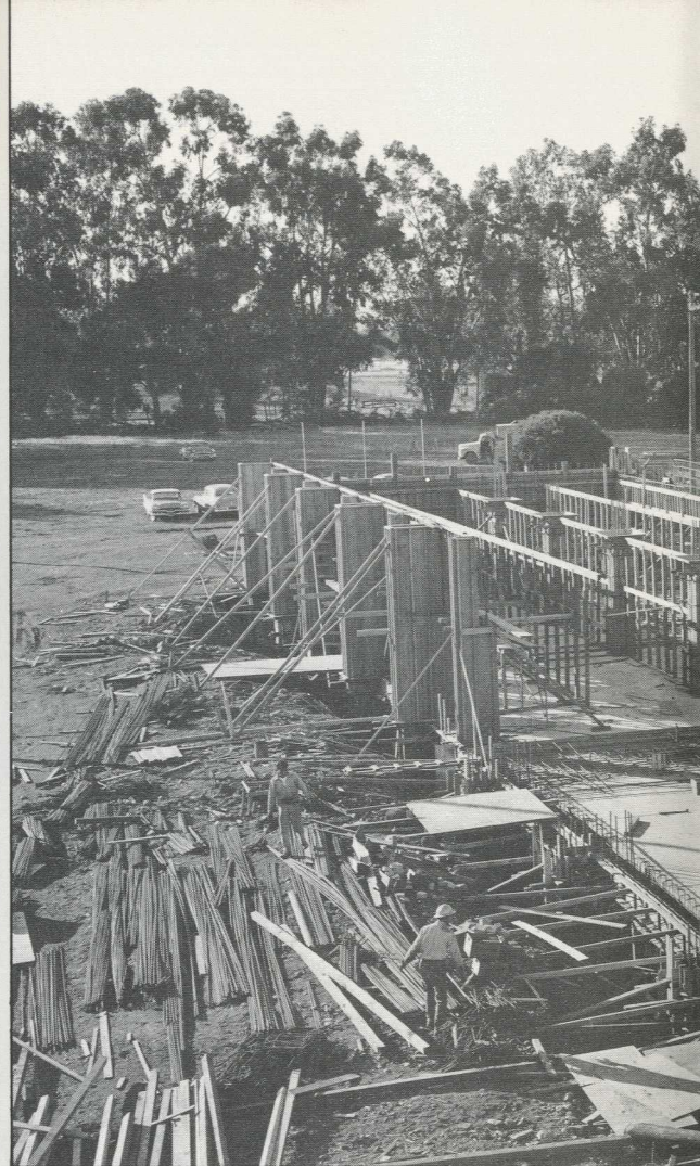
Medical center construction began in 1957 and was completed in 1959. The formative stages of the hospital's east wing with core building can be seen.
