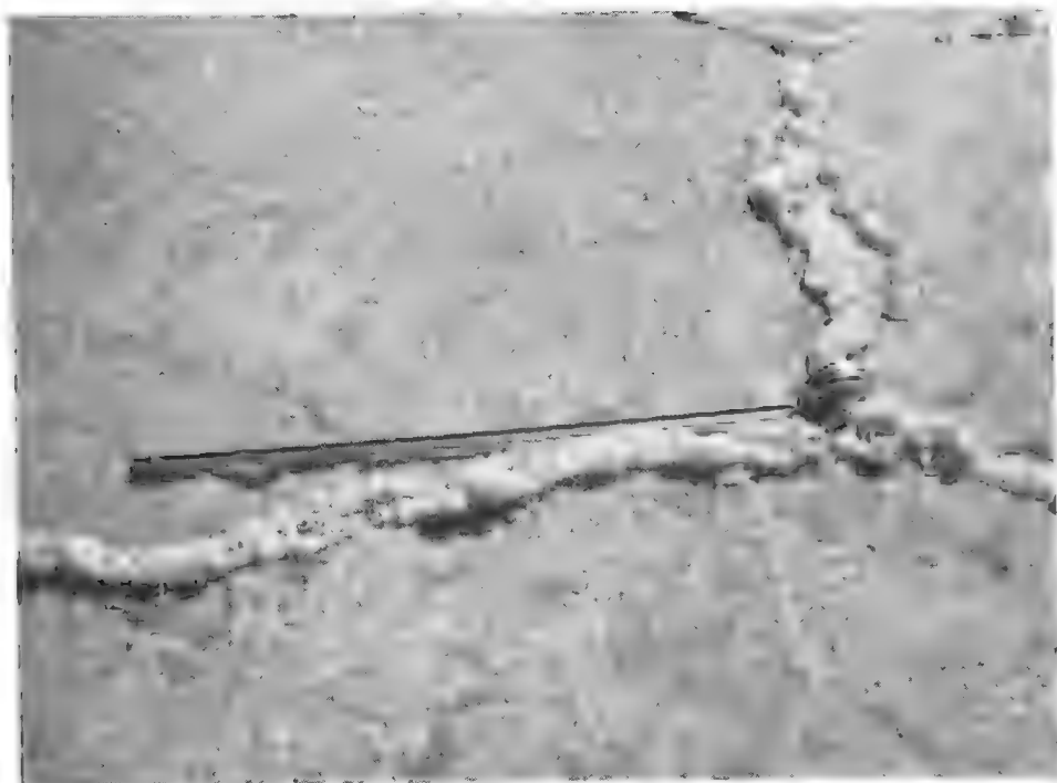
Fig. 1.—Efflorescent salt bulging from cracks in crust. (18-in. of tape measure gives scale.)
