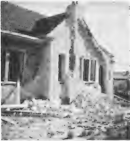
Stone veneer house in Aboyne Ave., Seacombe Park, showing damaged front.
