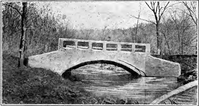
Fig. 98. A concrete bridge which failed on account of the foundation.
