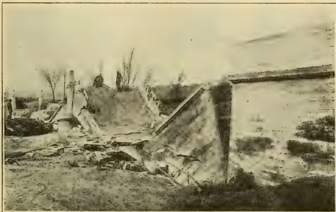
A so-called permanent patented reinforced concrete arch bridge after six months' use. The structure was 250 feet long.
