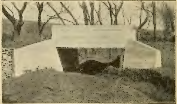
A concrete culvert. This culvert in Wabaunsee county will require no repairs and will last forever.
