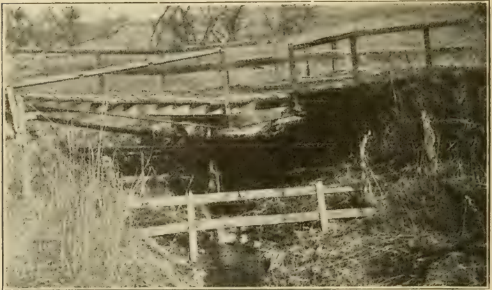
One of the most dangerous and most inexcusable places in the road.
