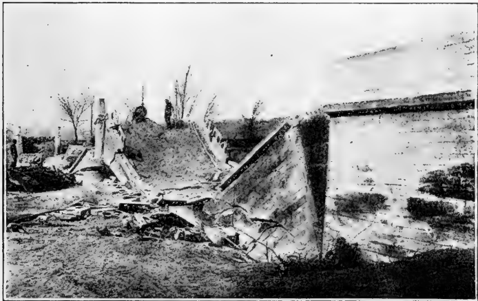
A so-called permanent patented reinforced concrete arch bridge after six months' use. The structure was 250 feet long.
