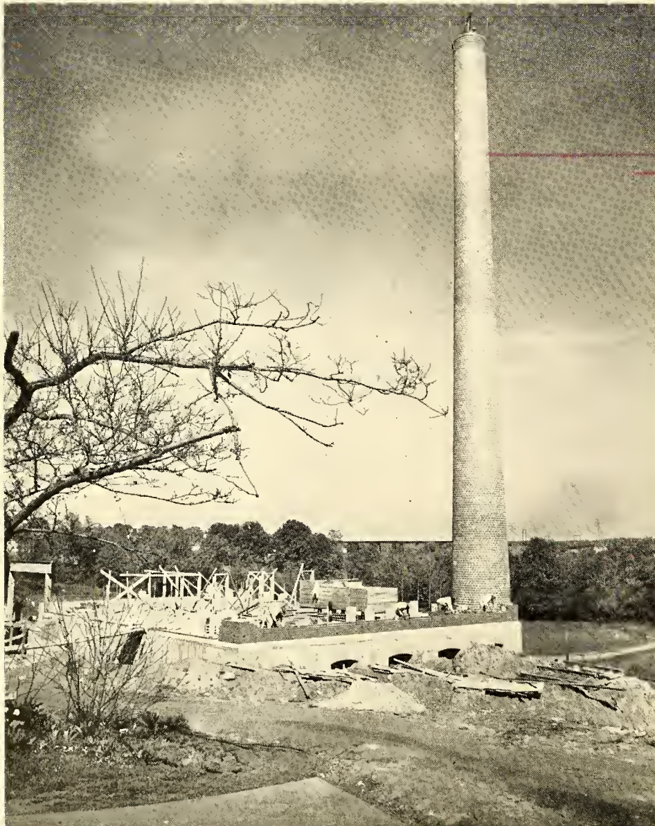
Salem's new steam plant is expected to be in use this summer. It will also house the laundry, shops and garage.
