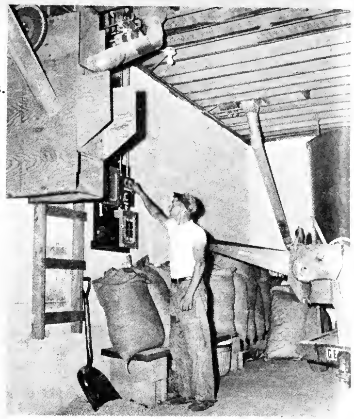
Jim Barbour installed time clock controls on augers discharging into pipes from overhead bins.
