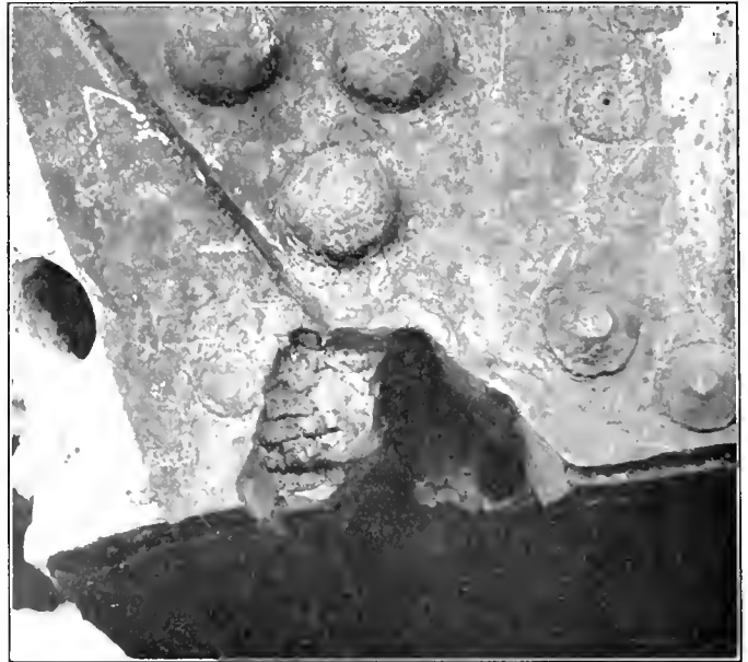
Fig. 2—It Was Necessary to Remove More of the Defective Mud Ring After Being Partially Welded.
