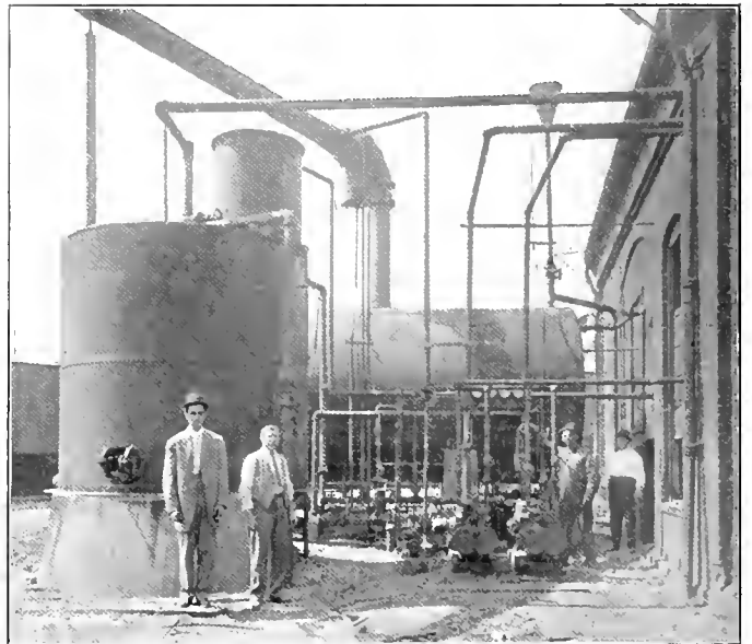
Boiler Washing and Refilling System.
