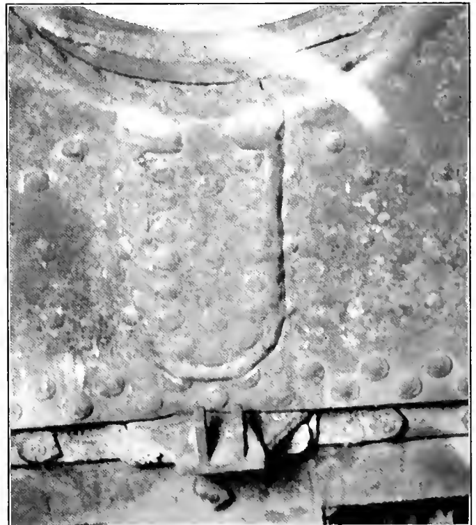
Fig. 5—Patch Under Fire Door with Edges Welded Instead of Calked.
