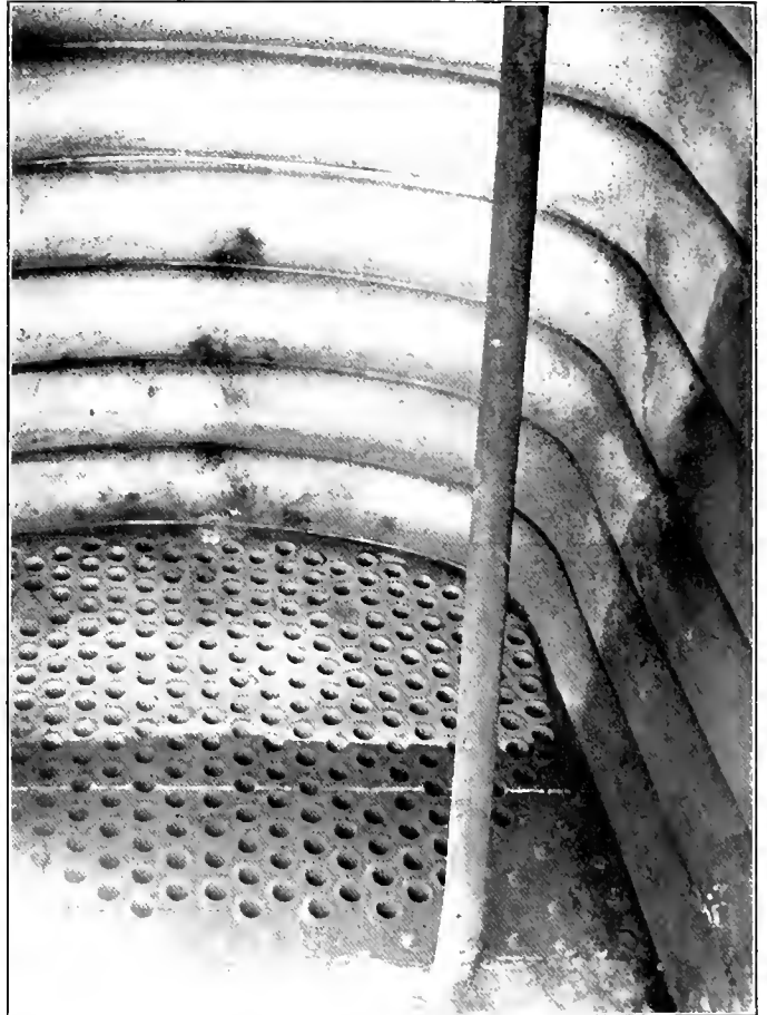
Interior of the Jacobs-Shupert Firebox After the Low Water Test.
