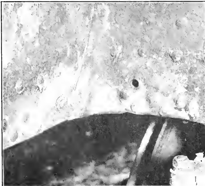
Fig. 4—Showing the Inside of the Firebox Where the Mud Ring Was Welded.
