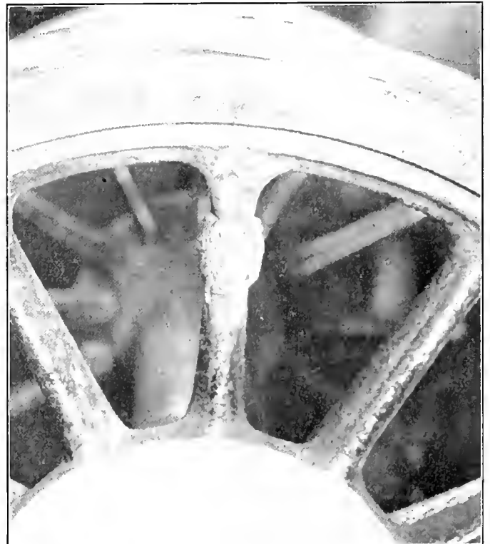
Fig. 15—Trailer Wheel Spoke Welded But Not Dressed.
