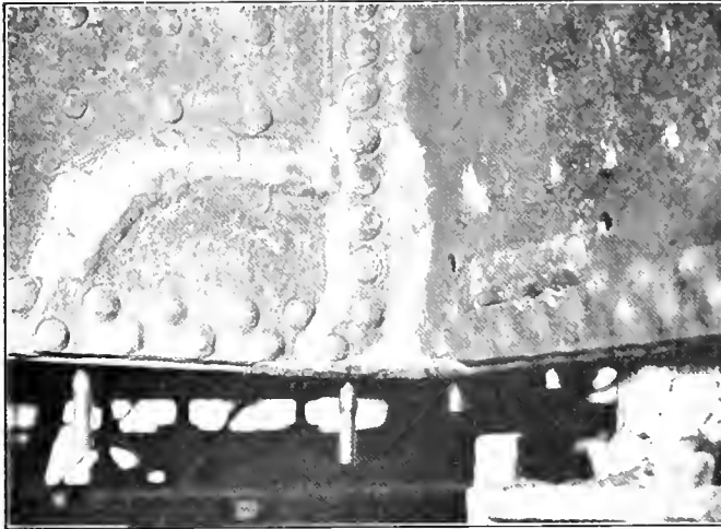
Fig. 9—Electrically Welded Crack in Corner of Firebox.
