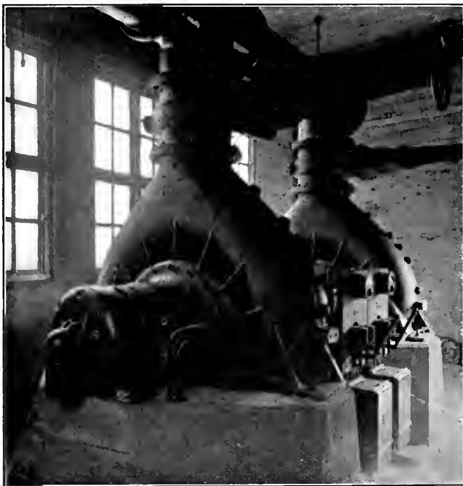
Blowers in Gas House.
