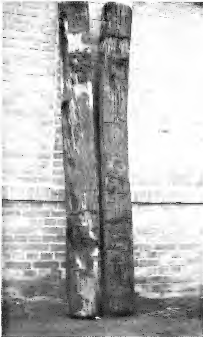
PINE TIES TAKEN FROM TRACKS OF PRUSSIAN STATE RAILWAY AFTER TWENTY-THREE YEARS' SERVICE. TREATED WITH ZINC CHLORIDE AND CREOSOTE.
