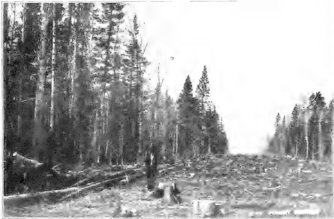
CLEARING RIGHT OF WAY FOR RAILROAD THROUGH DENSE TIMBER—SLASH BURNED CLEAN UNDER DIRECTION OF RANGER—PULP WOOD WILL BE HAULED OFF.
