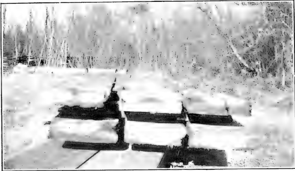
DECK PLAN REPLACED BECAUSE OF DECAY.
