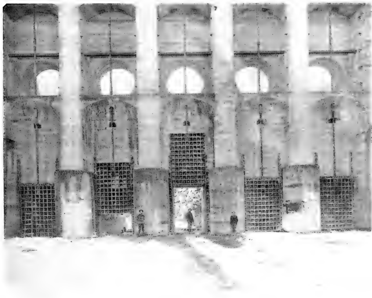
View showing five Coffin 8x12 regulating gates, Diversion Channel, Minidoka Dam, Idaho.
