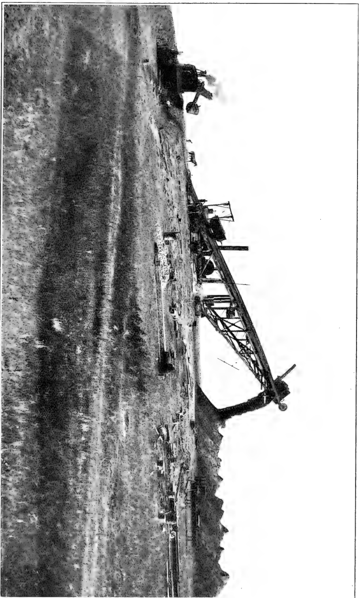
Steam Shovel and Derrick Cars in operation on Belle Fourche Project, South Dakota
