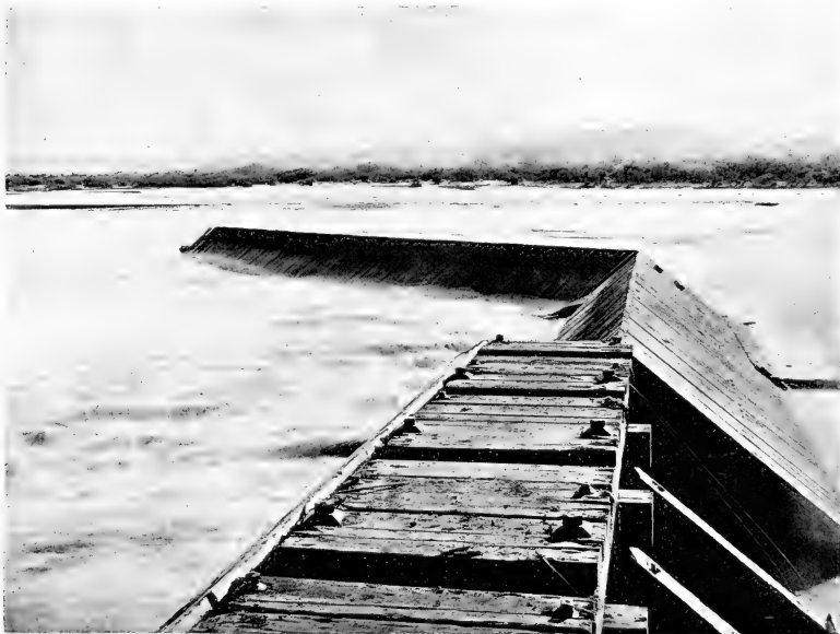
View Showing the Remaining Portion of the Arizona Dam, which was Washed Away by the Flood of April 13, 1905.
