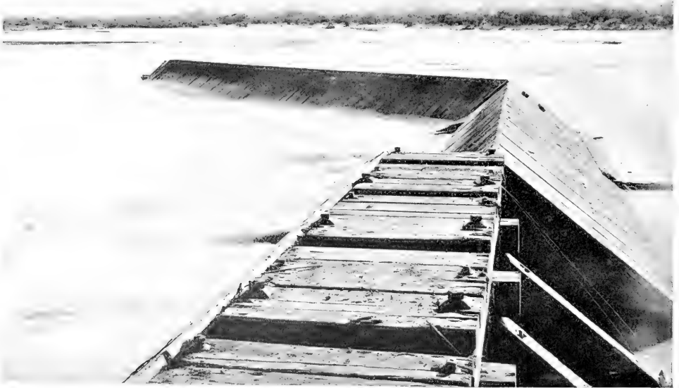
View Showing the Remaining Portion of the Arizona Dam, Which Was Washed Away by Flood
