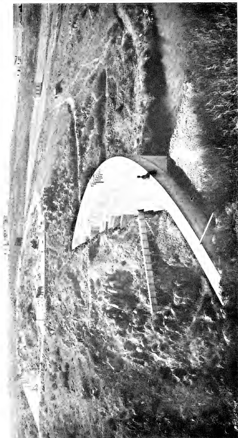
Upper Dam on Ouy Creek, near San Diego, Cal., Looking across the Canyon. This and the Sweetwater and Bear Valley Dams, All in Southern California, Are Curved with Arch Upstream
