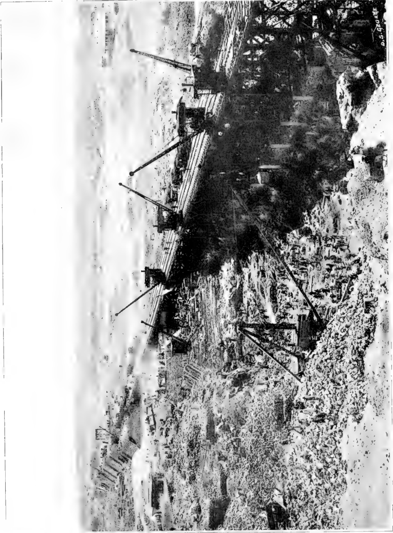
The Assouan Dam in Course of Construction. Filling in the Excavations with Masonry
