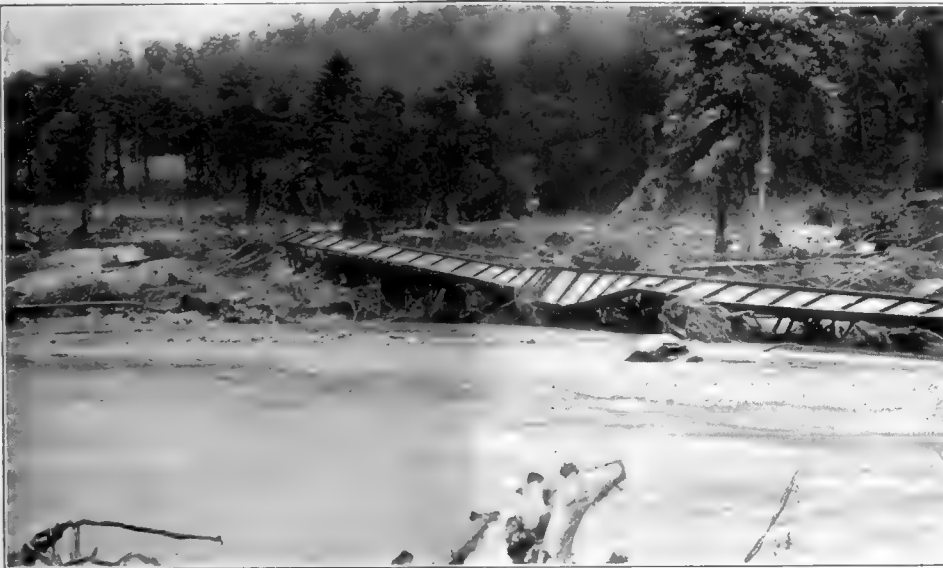
IRON GIRDERS CARRIED AWAY BY FLOOD
