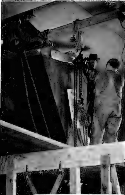
Working close under the ceiling to put in place again by the help of tackle one of the removed pieces, nearly a ton in weight
