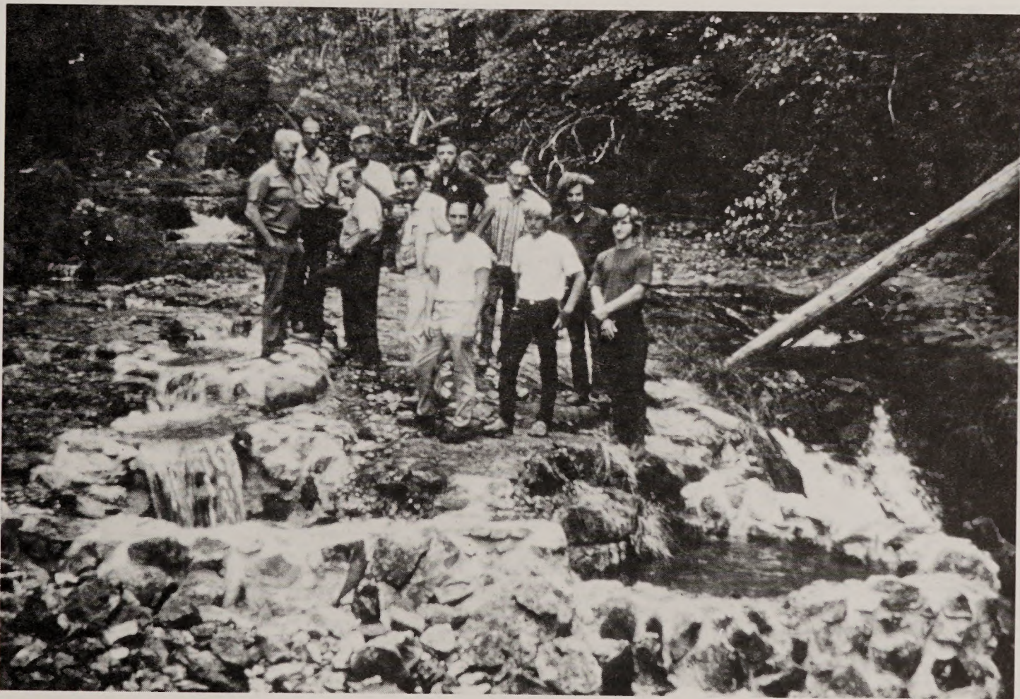
7. Volunteers stand by a series of jump pools they helped construct which will allow adult salmon to negotiate waterfalls and reach spawning areas upstream.
