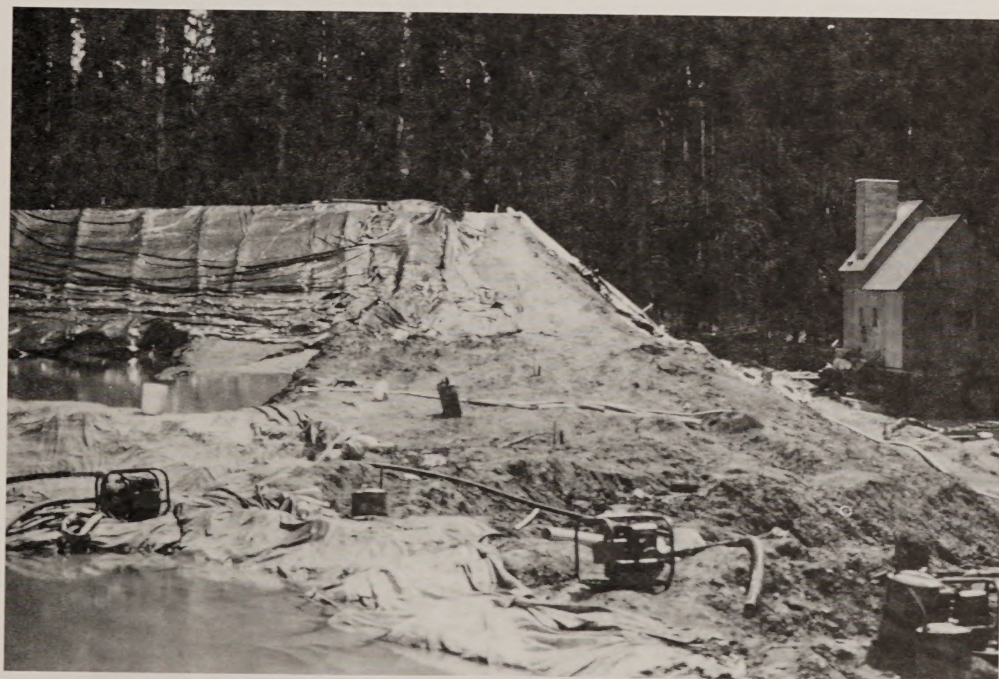
11. Gold heap-leaching processing adjacent to an anadromous fish stream is subject to cyanide leakage.
