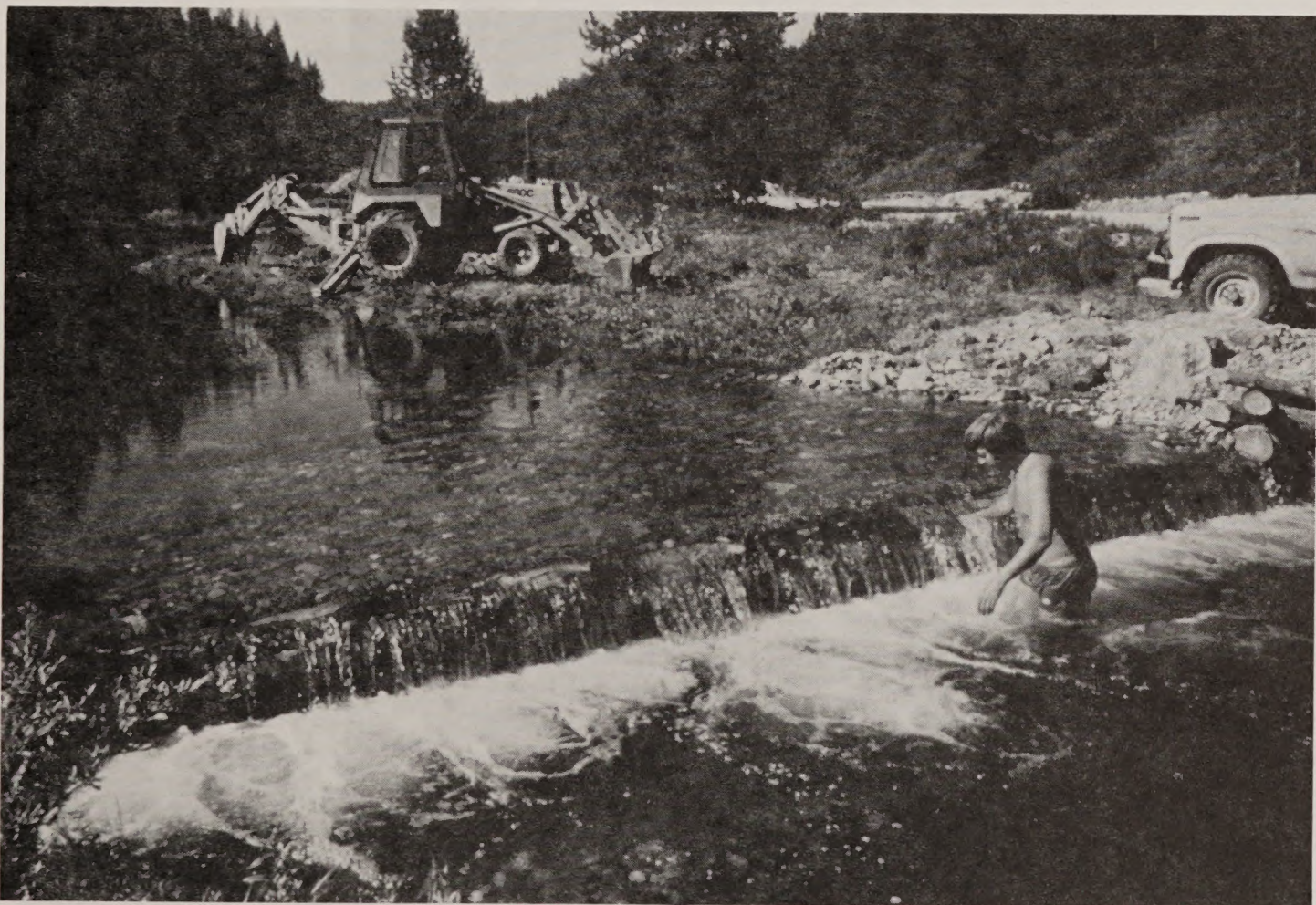
4. Completed "K" dam creates a spawning area above and excellent pool habitat below the dam.
