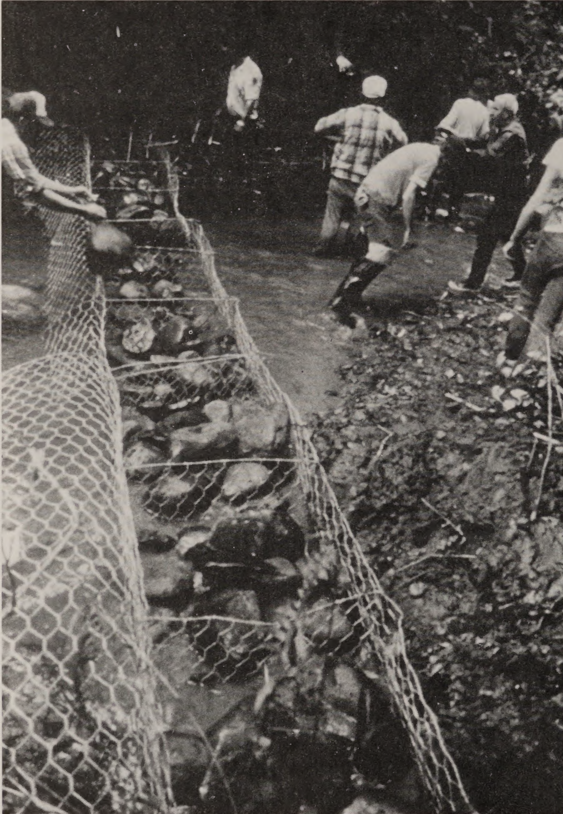
5. Volunteers fill wire gabion baskets with rocks used to create pool and spawning habitats and protect streambanks.
