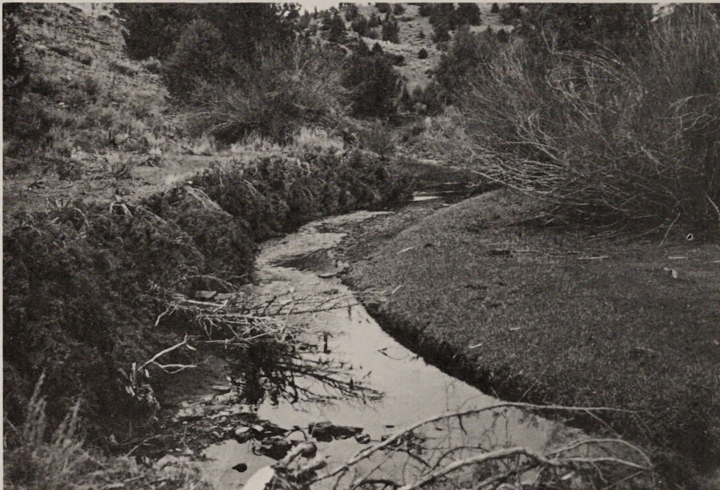
2. Juniper trees are cabled along damaged streambanks to trap sediments and provide cover for fish.
