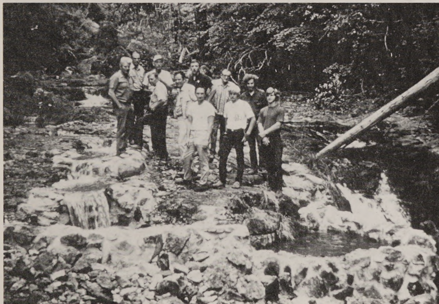
7. Volunteers stand by a series of jump pools they helped construct which will allow adult salmon to negotiate waterfalls and reach spawning areas upstream.
