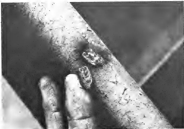
Figure 12. Area shown in Figure II with rust removed.
