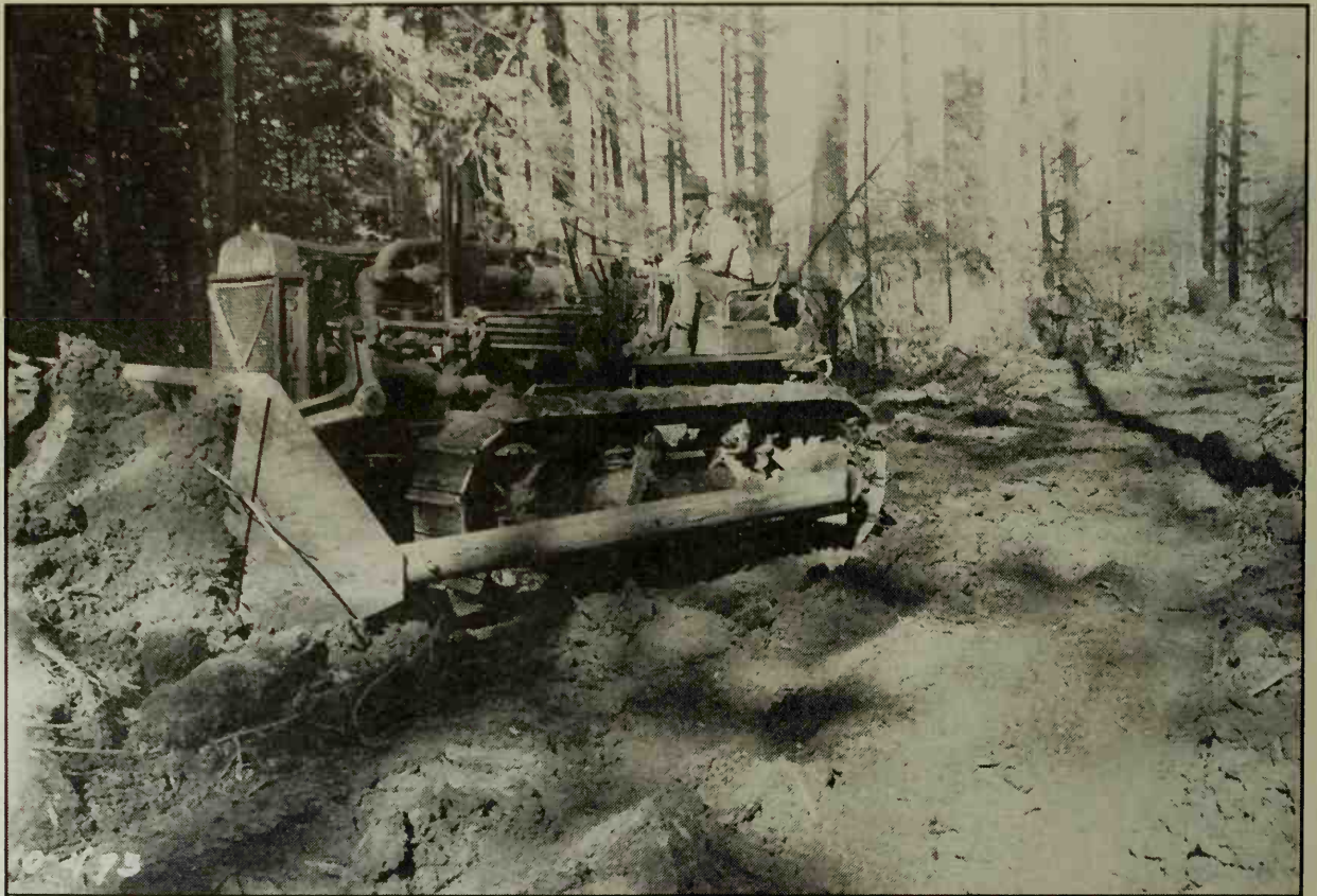
FIG. 45—THE "BULL-DOZER" AT WORK. GRADING IS PERFORMED MOST EFFICIENTLY BY WORKING DOWNHILL
