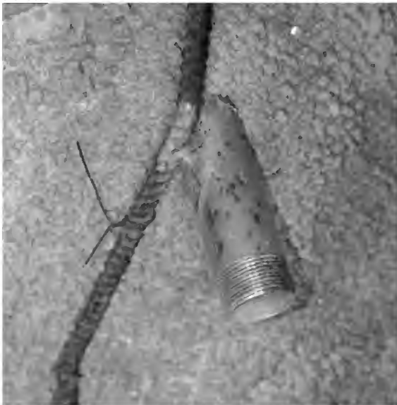
Figure 6: The amount of cement (or mortar mix) that goes through the diamond mesh and then seals to itself. This view includes the metal nipple welded onto the rebar.
