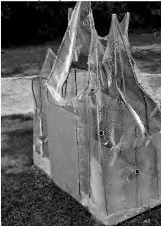
Figure 7. Finished view of metal portion of the mound: notice the bottom and back where we began adding the QUIKRETE®.
