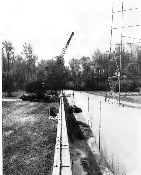
FIGURE 13. VIEW ALONG 635-FOOT TANK-(AN ENDOLOADER FOR MOVING SAND BEING LOWERED INTO THE TANK)
