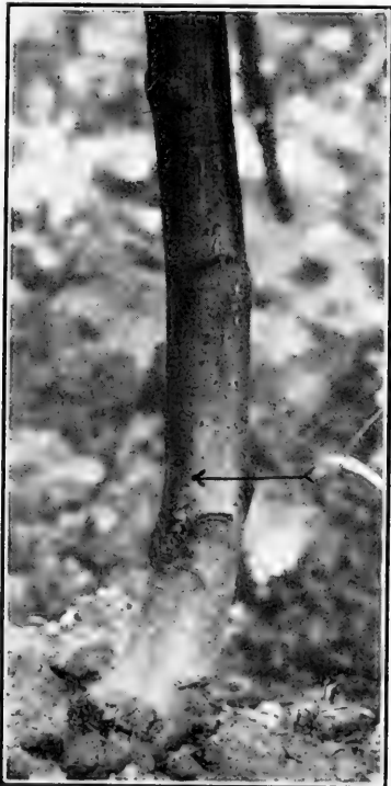
Note work of borer just where treatment with carbolineum ends. Shown by arrow.
