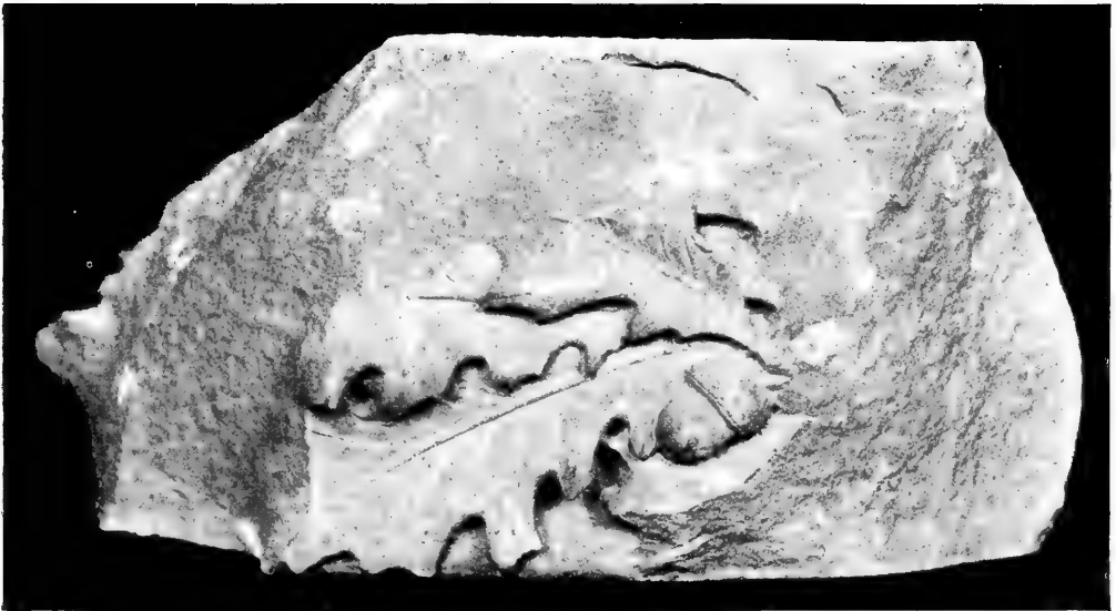
Effects of fire upon building stone. Above are shown spalls of granite from a column, below a cracked and broken sandstone cap; both are from the State Capitol, Albany, after the fire of March 29, 1911.
