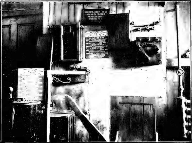
1. MILL SWITCH BOARD, SHOWING METHOD OF MARKING ELECTRICAL EQUIPMENT.
