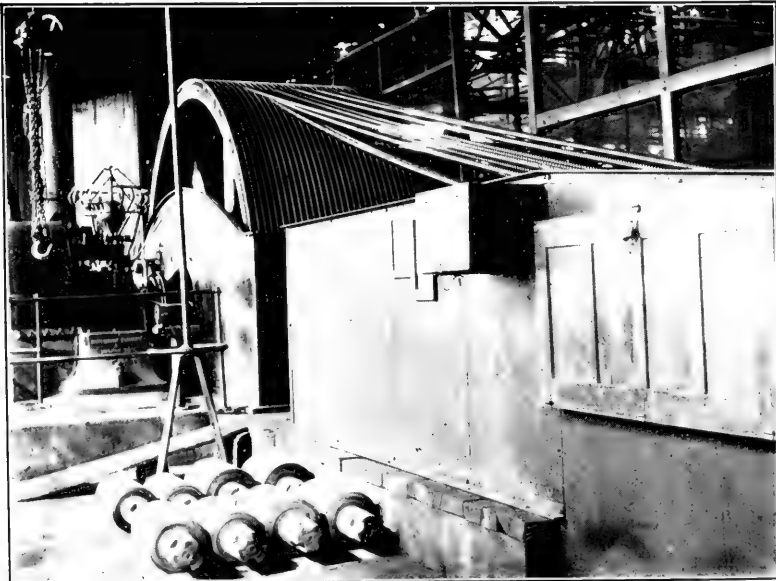
3. VIEW OF ROPE DRIVE FOR ROD MILL, SHOWING STEEL PLATE INCLOSURE.
