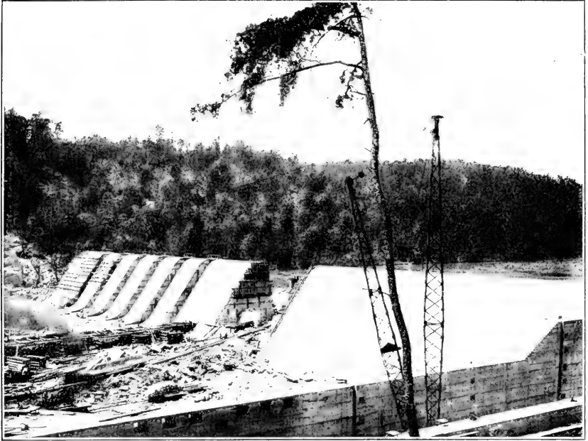
1. DAM NO. 17, BLACK WARRIOR RIVER, ALA., UNDER CONSTRUCTION. THIS DAM HAS A 63-FOOT LIFT, AND IS BEING BUILT BY PRIVATE ENTERPRISE FOR THE CREATION OF ELECTRIC POWER. LOOKING TOWARD THE ABUTMENT END FROM THE LOCK SIDE.
