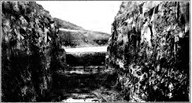
2. EXCAVATION FOR A LOCK IN THE BASALTIC ROCK FOR THE DALLES-CELILO CANAL, COLUMBIA RIVER, OREG.
