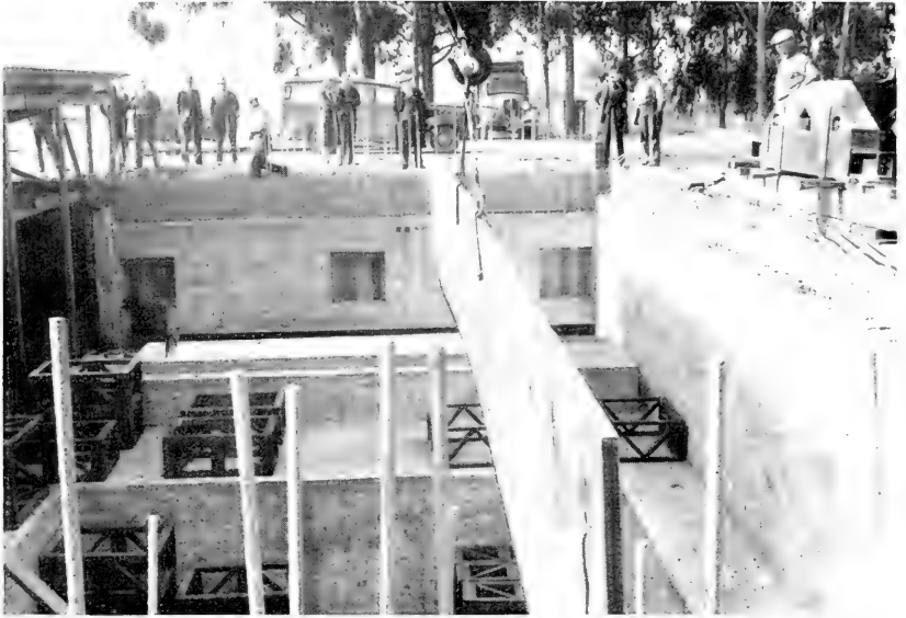
1. The first base plate being placed on the concrete foundation. The plate is 52 feet long, 75 inches wide, and 2 inches thick, and weighs 13\frac{1}{2} tons. There is about 1,200 tons of reinforced concrete in the foundation.
