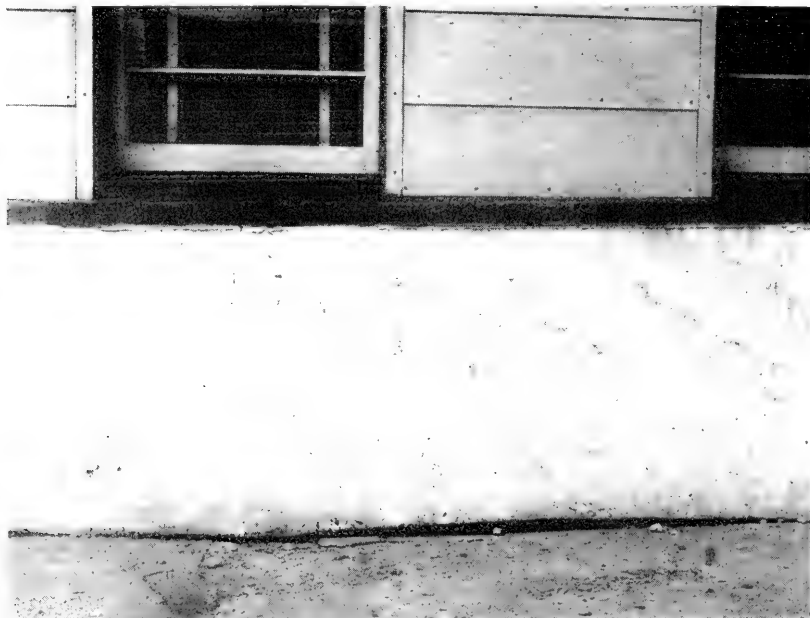
2. Settling cracks in foundation wall of the U. S. Post Office, Nome, Alaska, after thawing of permafrost under the building. Photographed August 10, 1948.
