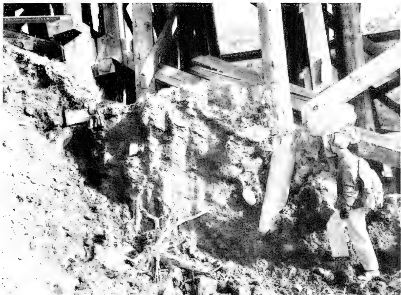
1. Bridge piling on the Alaska Railroad broken by downhill creep in mud on top of permafrost in the Nenana River Gorge, central Alaska. Photographed September 24, 1948.
