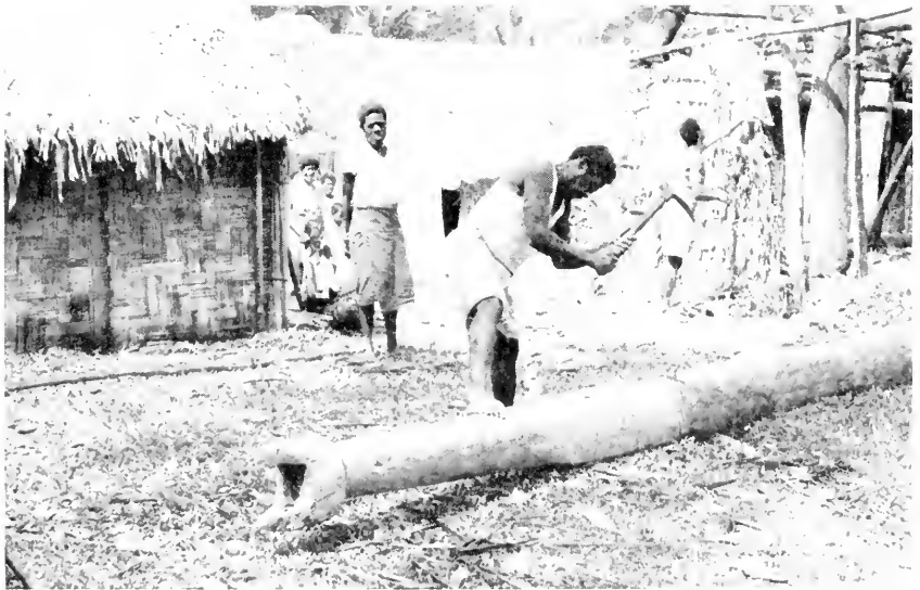
2. An upright for a house is shaped from a tree trunk with an adz. The usual tools for house building in Fiji are the machete, ax, and adz.
