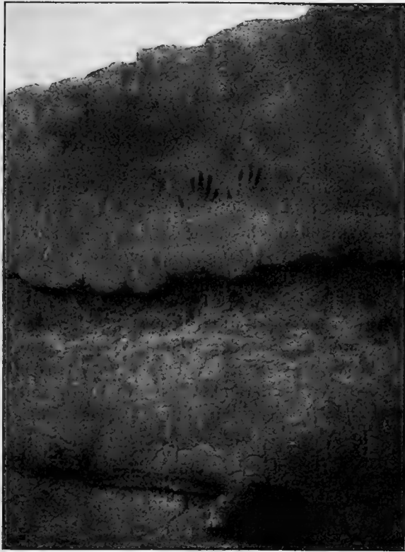
FIG. 16. Hand-prints and eroded base of wall of house in Compound D.
