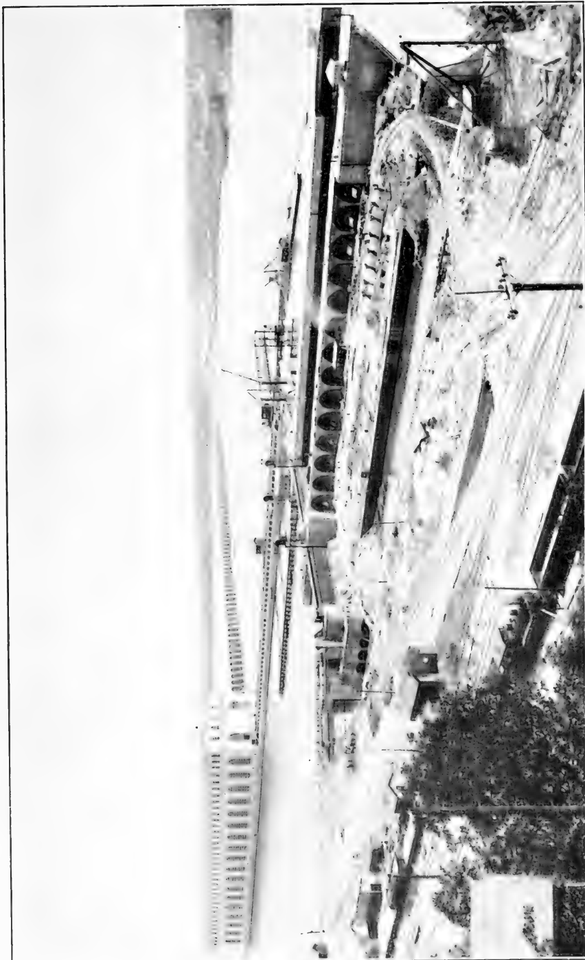
GENERAL VIEW OF THE WORKS OF THE KEOKUK-HAMILTON DAM FROM THE IOWA SHORE.
