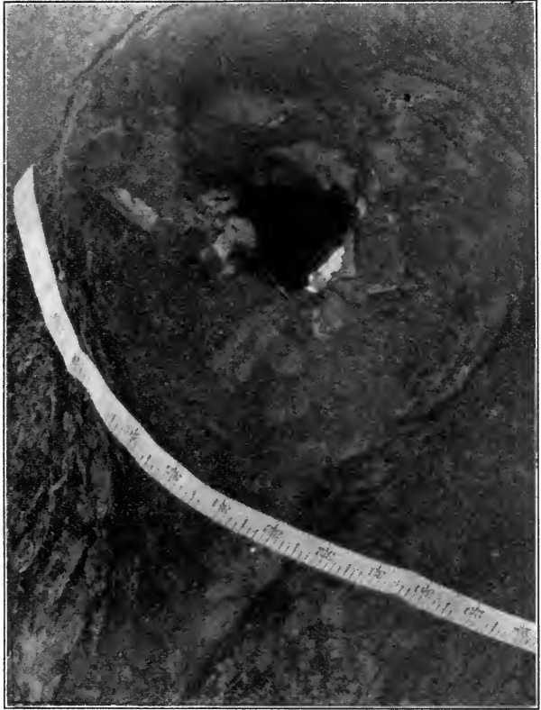
FIG. 50.—The decayed hole caused by wood-destroying fungi. (See Figs. 51 and 52.)
