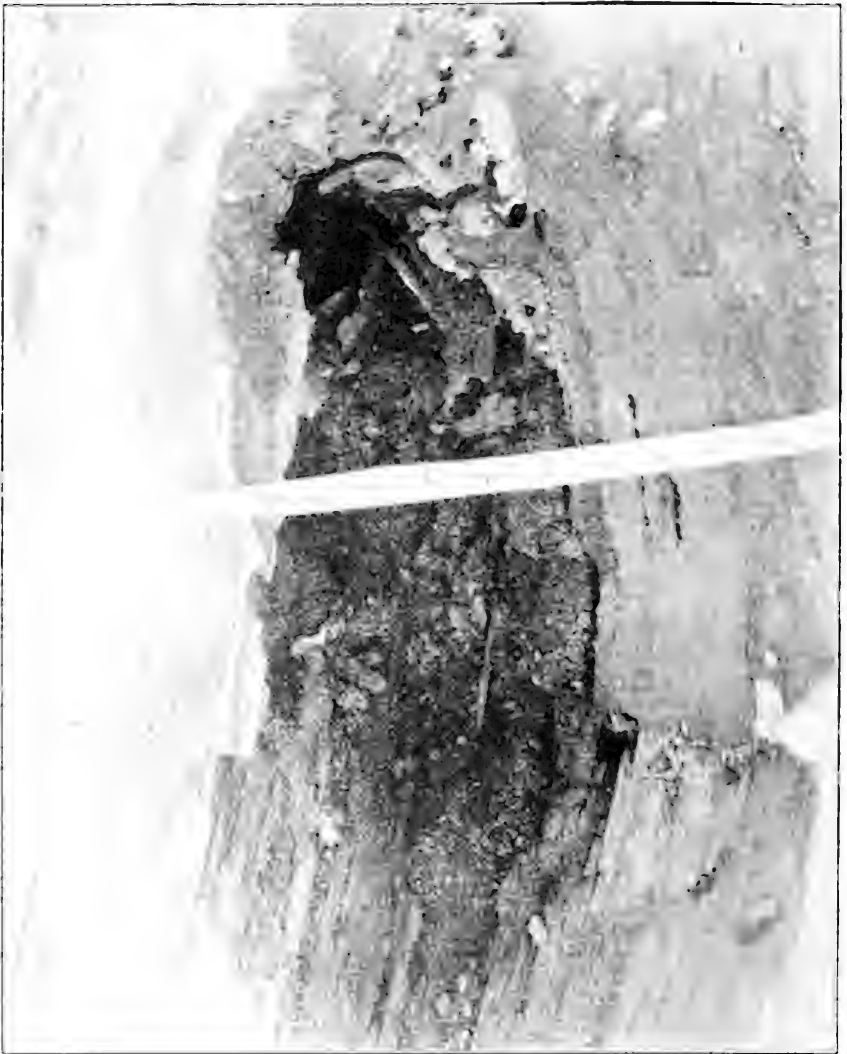
FIG. 51.—The same tree as Fig. 50, showing the extent of the decay. The tree was about 16 inches in diameter and had only about two inches of sound wood on the outside, a mere shell. The white mould is the mycelium of fungi.
