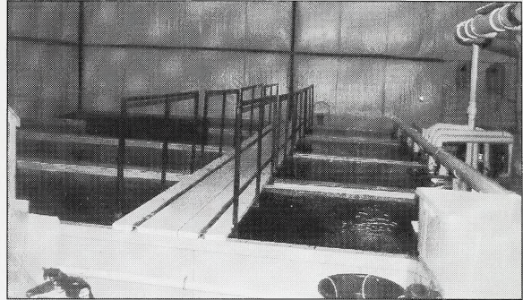
Ackenberry's indoor water recirculating trout rearing facility
