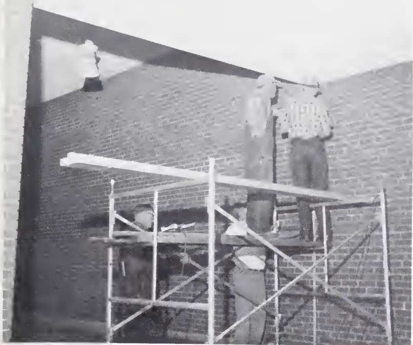
Workmen put up a partition in the North Hall to form music room.
